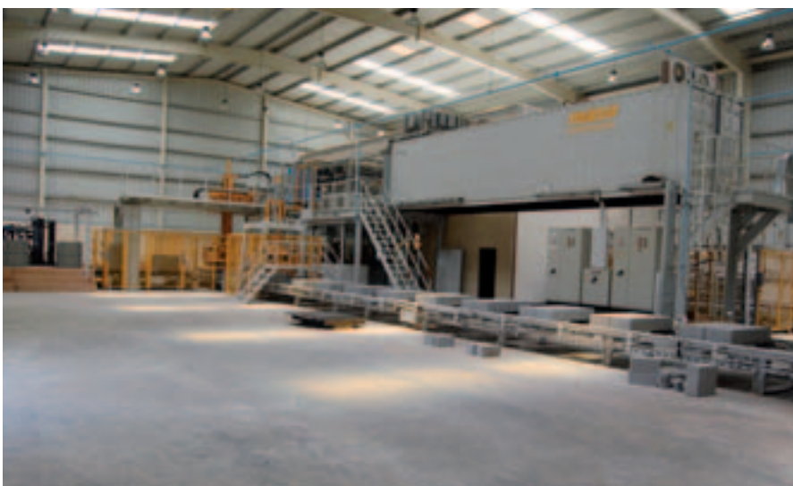
All of the electrical control cabinets for the entire block making plant are housed in a single container, which Masa calls the Powertainer.
